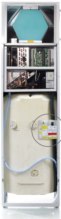
The button for the emergency operation are located behind the large door
